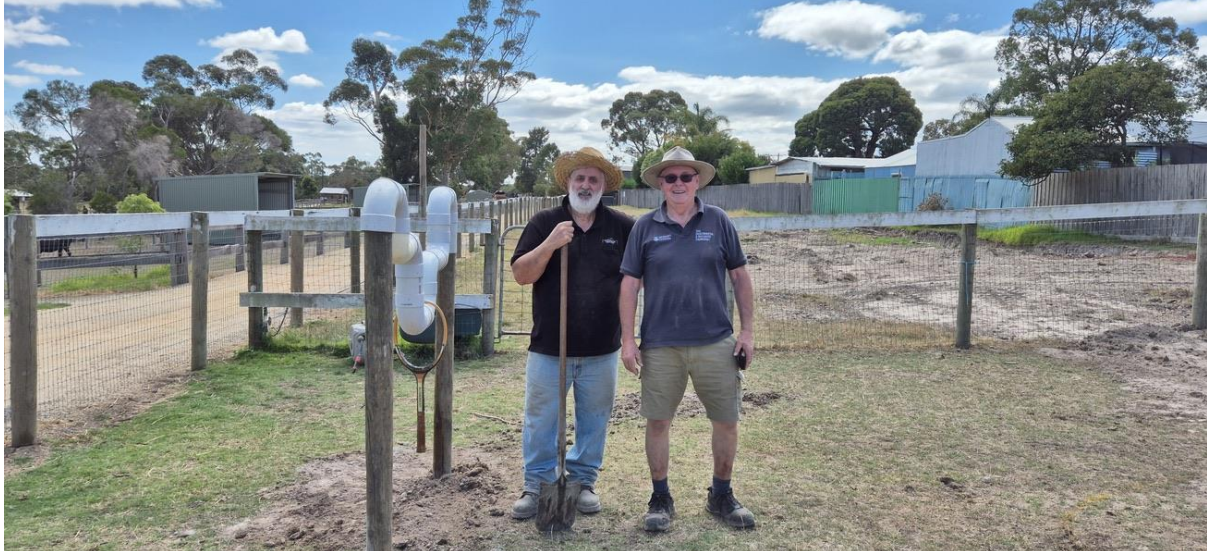
At Myuna farm on Wednesday, we started the on-site installation of the pony trial stations for children with disabilities
